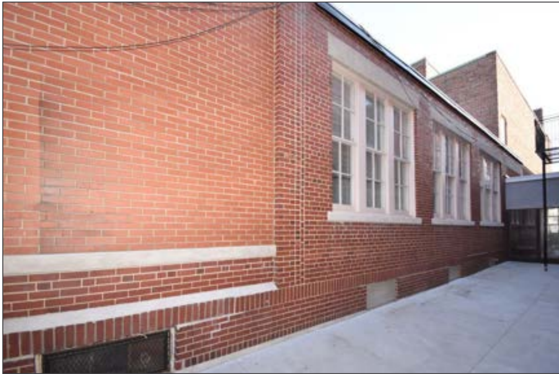
15. View looking east towards the Woonsocket Commercial School (foreground) and CYO passageway (far right) with Masonic Temple in background.
