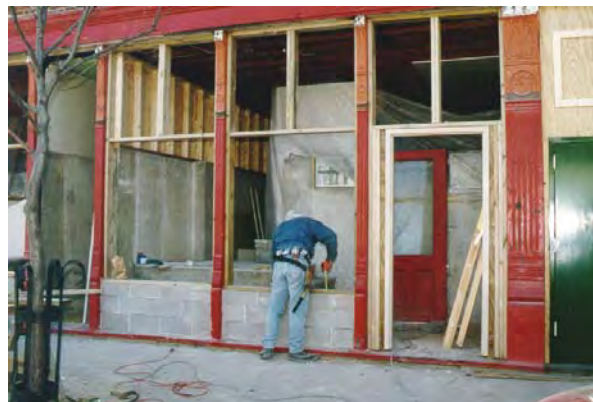
Floodproofing the vestibule of a storefront
