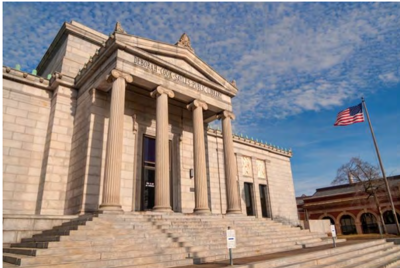
Figure 9: A 2019 CLG grant to the City of Pawtucket funded a professional Conditions Assessment of the Pawtucket Public Library's Sayles Building (1899).
