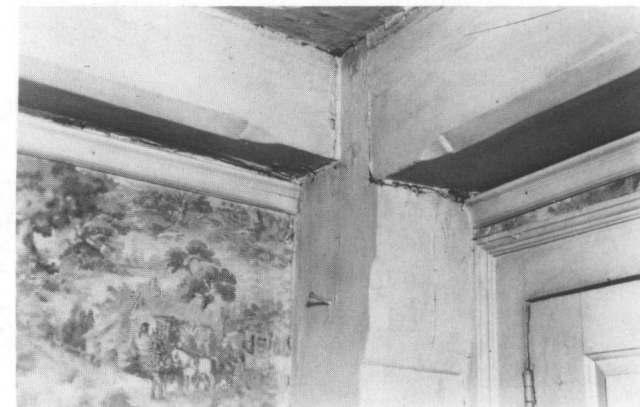
Fig. 6: Interior, Valentine Whitman, Jr., House (c. 1694); Great Road; photograph, 1937. Chamfered corner post and plates are shown.
