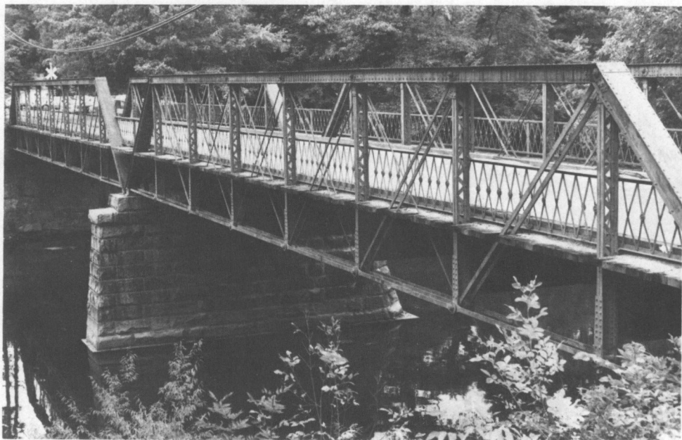
Fig. 33: Albion Bridge (1855). A Pratt pony-truss bridge, of pinned and rivetted construction, the Albion Bridge is composed of two 211-foot spans supported by a center granite pier.
