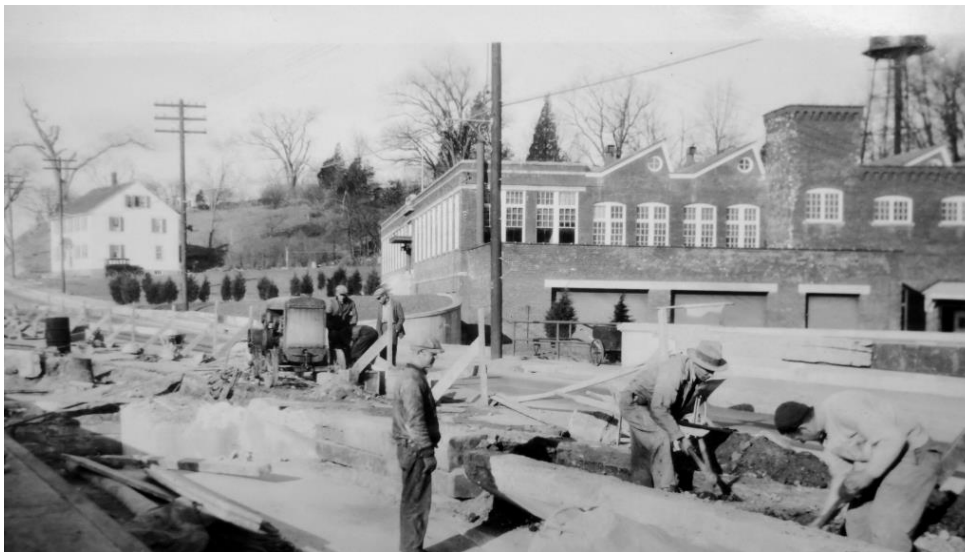
Figure 6 RI SBPR photo 108091 showing widening of Branch River Bridge No. 108 (December 1930). Former Andrews Mill office, weave shed and loading dock in background. The 2½-story residence in the rear left was a Pitts Mill worker tenement (demolished after 1949).
