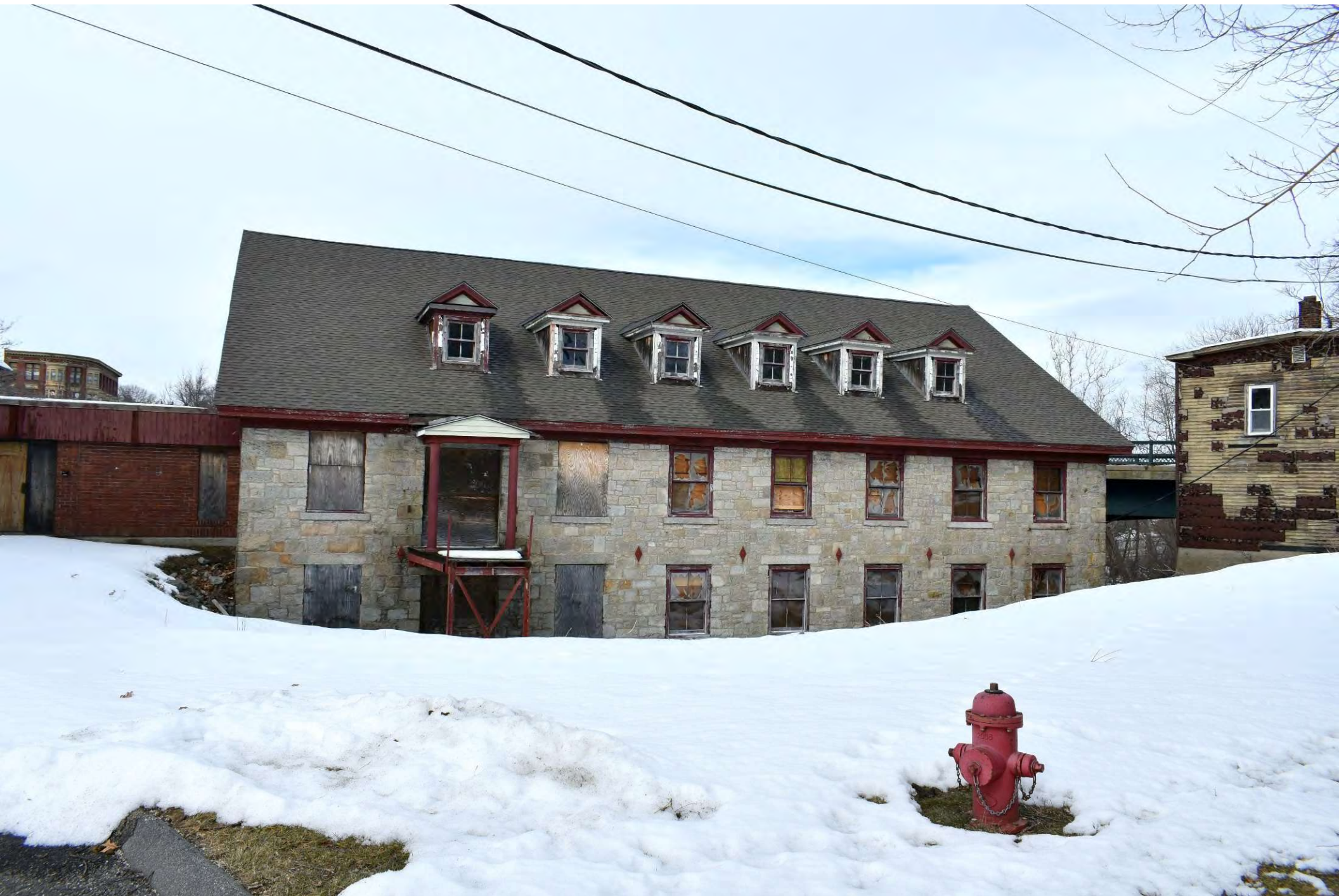
Photo 8 of 30: #4 Mill east elevation (left) and 125 Court Street south elevation (right), facing northwest
