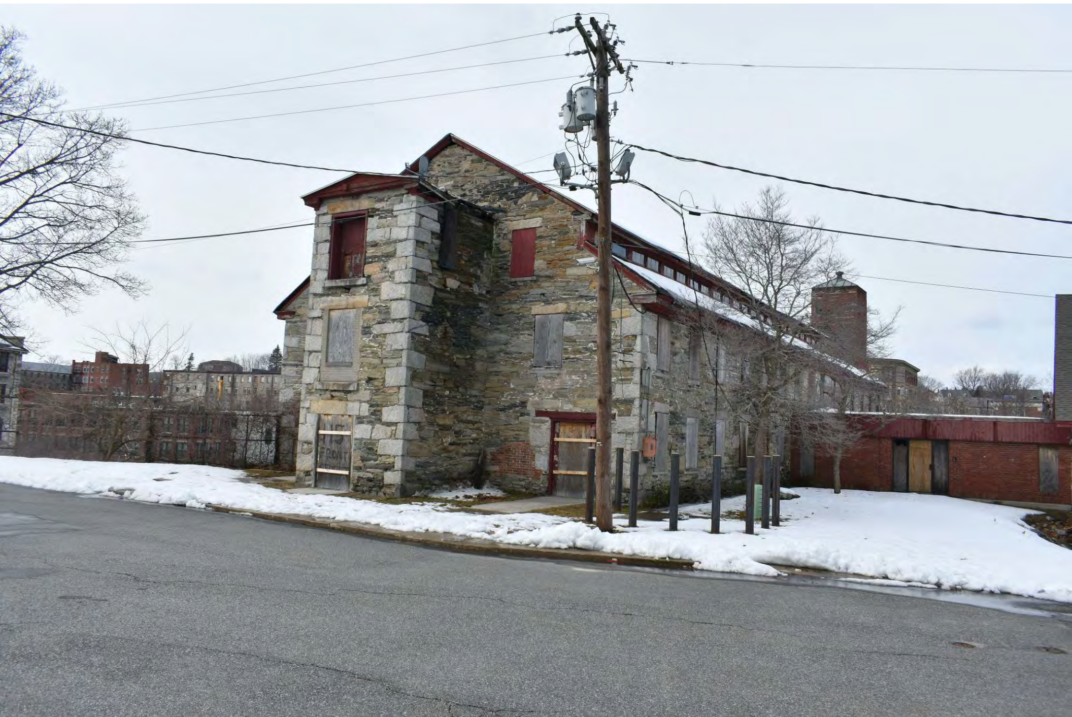
Photo 2 of 30: # 1 Mill, east and north elevations (left) and c.1980 brick connector (right), facing southwest
